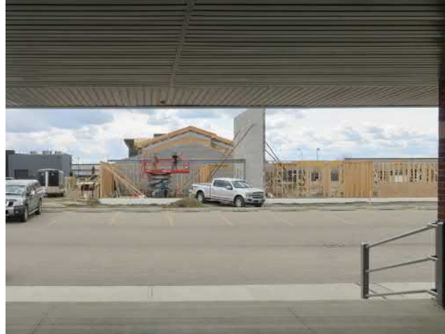
Sign of encroaching construction
