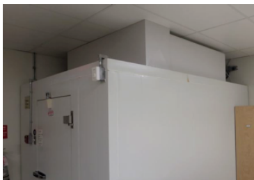
Note the shroud which encases the motor atop the cooler.
