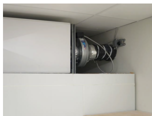
The installed fan ventilates the area via the vent to the outside.
