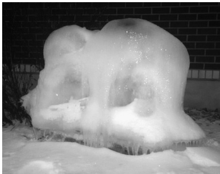
Steam emitted from the two temple boilers through two venting pipes under the eaves on the east side of the building condenses to water on cold days and drips to form layers of ice. The elephant look-alike was detected in the resulting ice sculpture. Photo: David Tanaka
